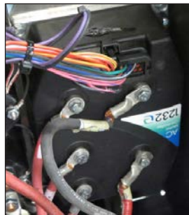
Figure 2: Wheel Drive Controller
